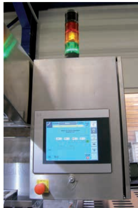
Opelka programmed the PLC and HMI applications entirely in B&R's Automation Studio engineering environment. The seamless integration made programming, diagnostics and maintenance remarkably efficient.
