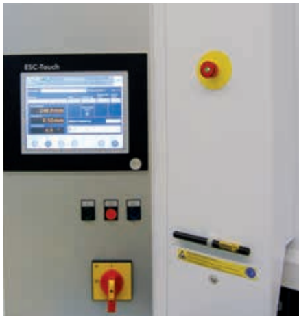
EHT's new ECS-Touch controller is based on a Power Panel 520 from B&R. In addition to controlling all of the machine's processes, it also serves as an HMI platform and operator interface.
