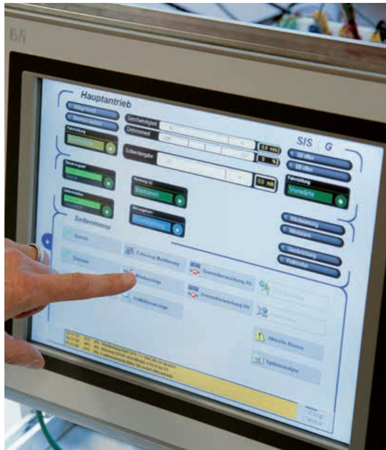
The new gondola lift at the Jakobshorn resort features a PLC, touch screen operator panels and frequency inverters from BSR.
