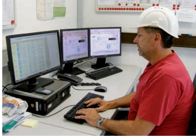
CHT's process sequences are much easier to analyze with APROL. TrendViewer and AuditTrail now permit analysis of processes that couldn't even be observed with previous solutions.
